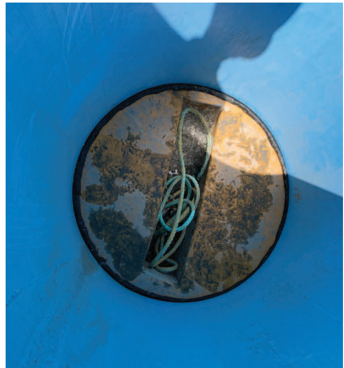
Ensure riser is sealed on FRP base liner joint, ensuring mastic sealant is fully engaged
