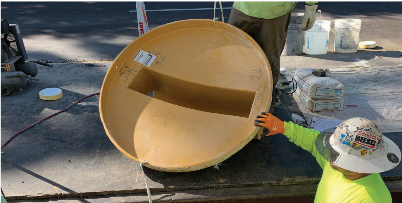
All components labeled
