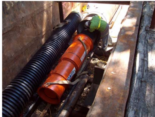
Figure 6: OSHA Approved Ventilation Equipment w/ Corrugated HDPE Ducts
