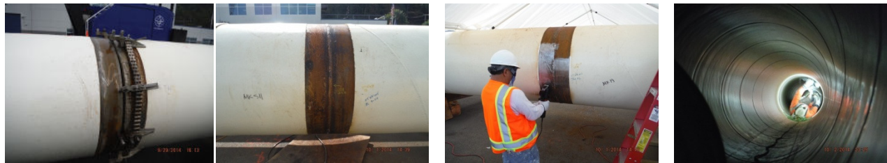
Figure 10a, b, c, d: Joint alignment for Butt Welding, Completed Butt-welded Joint; Surface Grinder Used for Substrate Preparation for External Joint Completion, Surface Preparation for Internal Joint Completion
