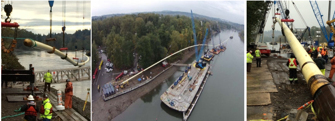
Figure 12a, b, c: Lineup of Pipe in Preparation for Pull-back; Complete Line Ready for Pull-back; Pull-back Commencement by Insertion into
