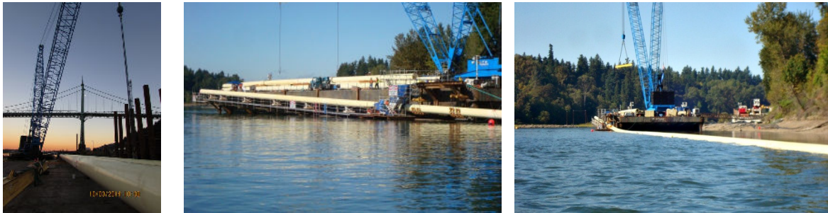
Figure 9a, b, c: 240-ft Welded Segment of Steel Pipe, Transportation of 240-ft sections by Derrick Barge, Final Joint Assembly Prior to Pull-in
