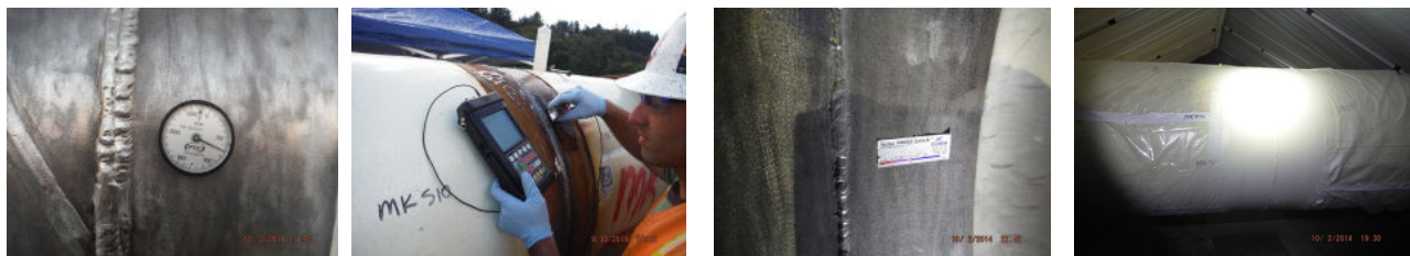
Figure 11a, b, c, d: Ambient Temperature Conditions, Surface Temperatures, Testex Tape for Anchor Profile Testing, Completed Joint Coating
