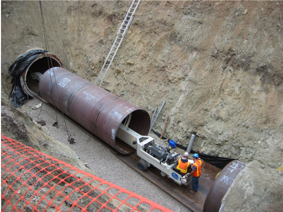
Figure 4. Pipe carrier a portal
